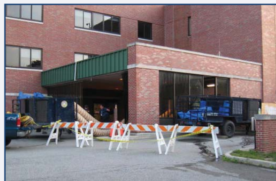
The ECU located on the DRASH UST Trailer (shown in front of the ER entrance) was used to cool and provide electricity to certain portions of the hospital's emergency area.
